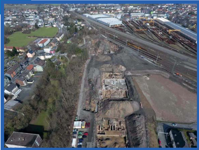
Drone photo of a commercial area in Witten with remains of Steinhauser Hütte during the excavation 2018 (© LWL-AfW/R. Klostermann)
