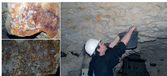
Salt Deposits on the chalky walls and the implementation of telltale plaster to supervise the stability of the structures, Spiennes, Belgium.
