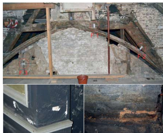
Crack measure apparatus set up on a half-timbered partition, the exfoliation of wall fillers and mortars further to an accumulation of salts, former monastic infirmary of the abbey Saint Jacques, Liège, Belgium.
